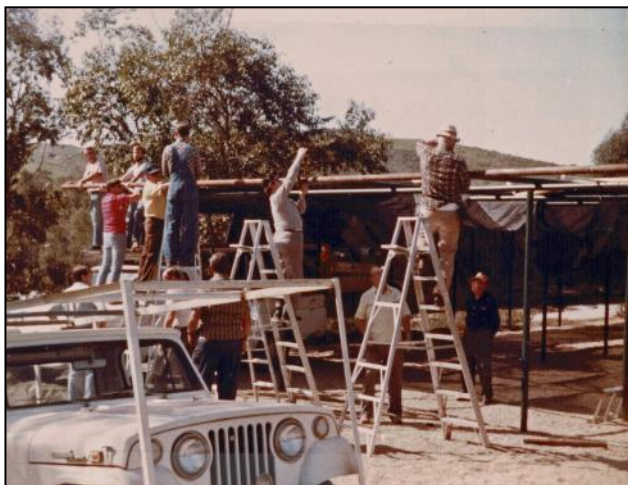
Putting up the "Front Porch" was Howard Jones, bossing from right to left Gene Lund, John Pilland, Vernon Hook, Dick Chadwick, Ed Broz, Gus Schlapfer, Bill Foster, Ray Conser, Ron Miller, Ed Post, and Nate Ogdon
